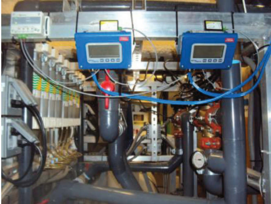
Figure 12. Ultrasonic Flow Meter Output and Data Logging System (Photo: Efficiency Solutions)
