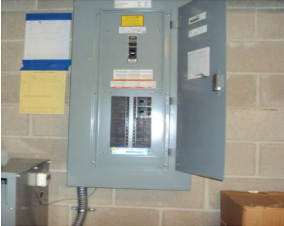
Figure 10. Installation of Watt Meter in Electrical Panel serving the AquaRecycle System (Photo: Efficiency Solutions)
