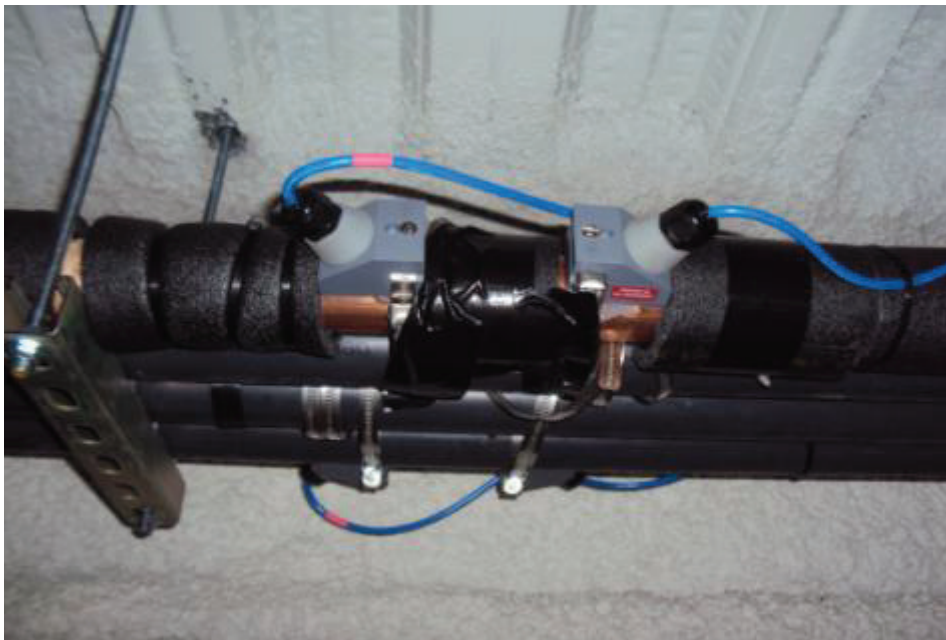
Figure 11. Ultrasonic Flow Meter as Installed on Recycled Water Piping (Photo: Efficiency Solutions)
