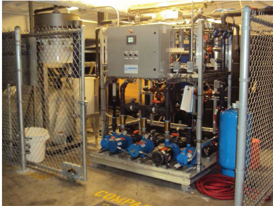
Figure 2. AquaRecycle System (Photo: PNNL)
