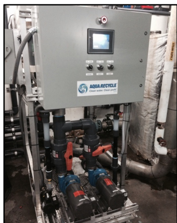
AquaRecycle's Control Panel at the Bonaventure.
